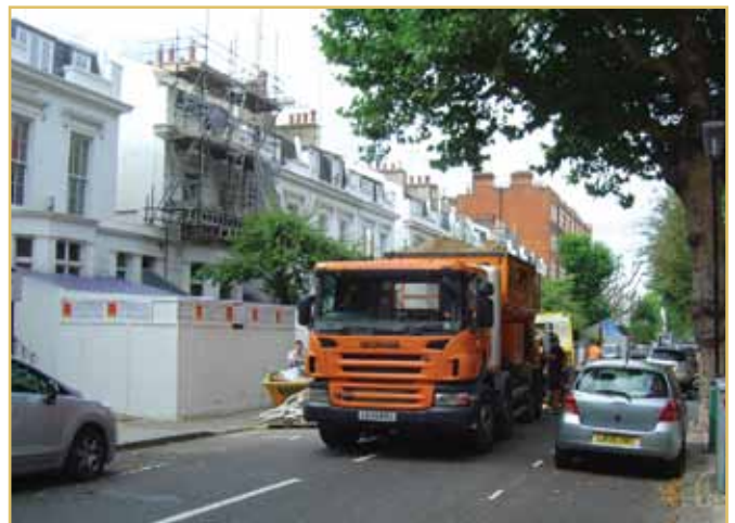
Despite the contractors assertions lorries block the road outside this subterranean development sometimes for a whole day
